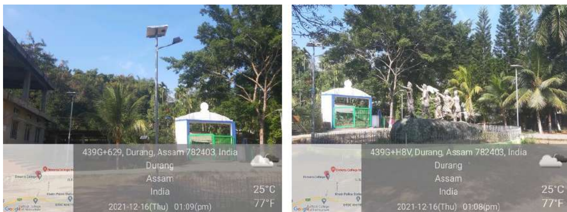
Figure 7: Solar Lights installed in the College Campus (sponsored by Star Cement under CSR Programme)
